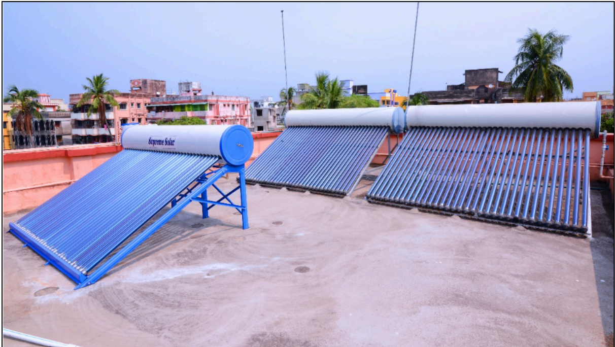
Supreme Solar Water Heater set up on 'Brahmananda Bhavan'
