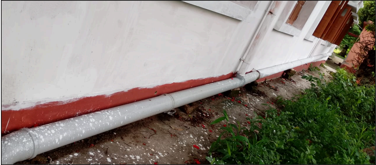
Pipe lines using rain water
