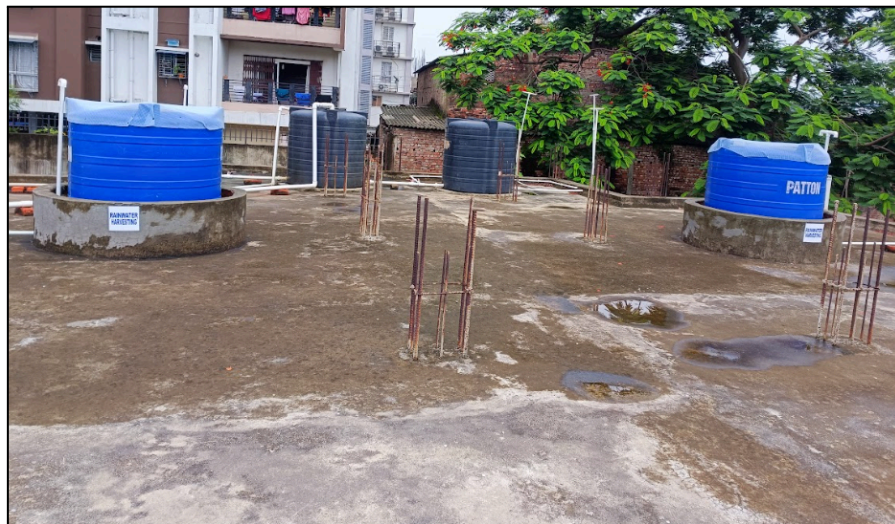
Pipe line fitted with the tank, collecting rainwater
